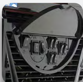
Panel de control.
