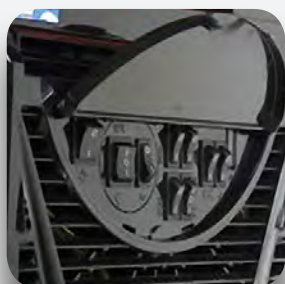
Panel de control.
